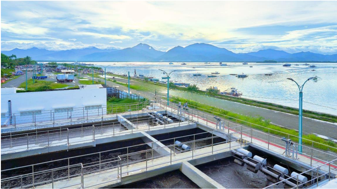
Puerto Princesa Water Reclamation and Learning Center, Inc. (PPWRLC), a 2MLD wastewater plant serving as the water systems enhancement infrastructure of Puerto Princesa, Palawan.
